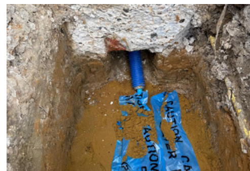
Pipe entering property through duct
