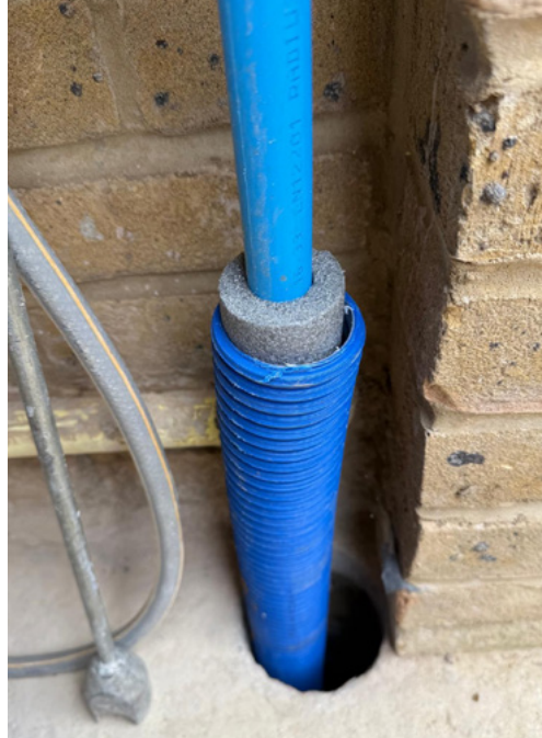
Ducting and insulation
